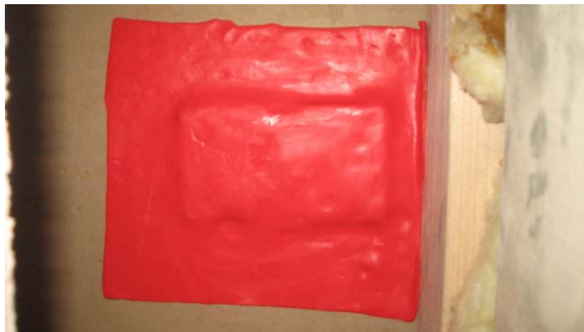
Figure 5 Putty Pad installed outside switch box
